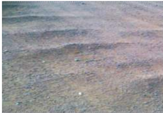
Photo 7.4.3 Corrugation of Bituminous Surface
