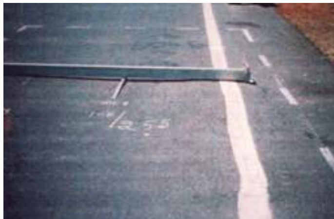
Photo 7.4.5 Shallow Depression in Bituminous Surface
