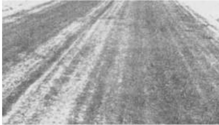
Photo 7.2.3 Streaking of Bituminous Pavement
