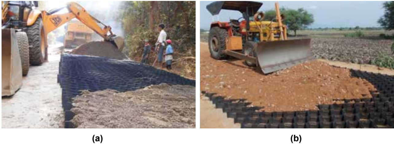
Fig. 6.6 (a) In Filling from Side, (b) Equipment Run on Geocell Filled with Soil
