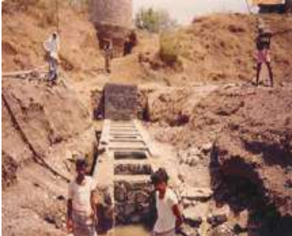
Figure 10.23: Horizontal Flow Filters
