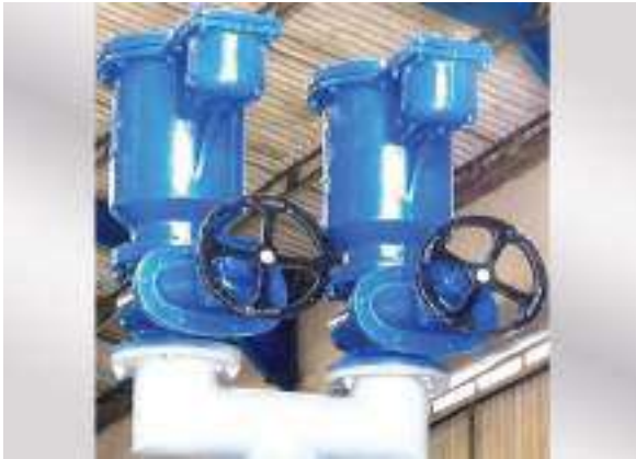
Figure 11.80: Double Chamber Kinetic Air Valve (Onsite)
