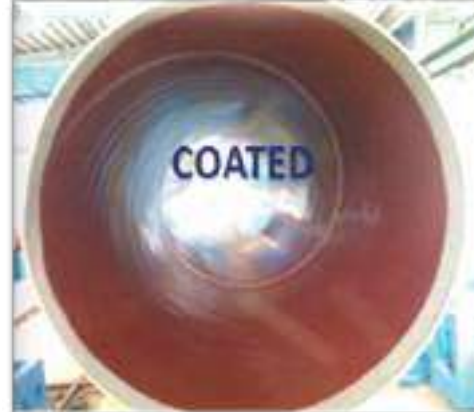
Figure 11.11: Internal Food Grade Solvent-Free Epoxy coating
