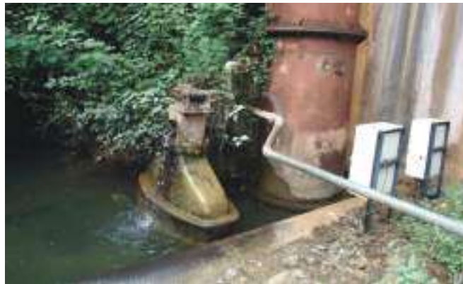
Figure 2: Leaking valve identified as a very high risk during WSP preparation
