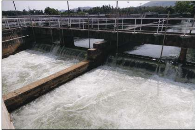
Figure 8.2: Weir Mixer (Rapid Mix Unit)
