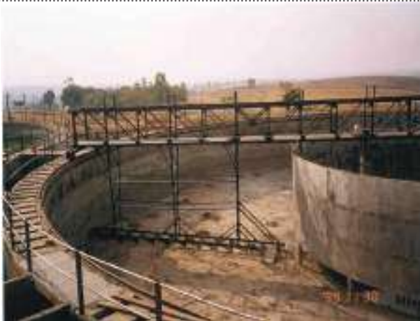
Figure 8.17: Clarification zone with scrapper rotating bridge
