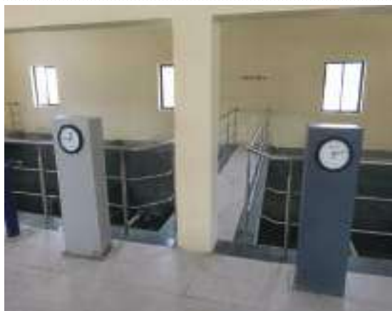
Figure 8.37: Rate of Flow and Head Loss Indicator (Mechanical)
