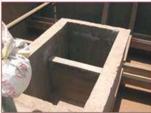
Figure 8.46: Close-up of Splitter Weir and Chamber
