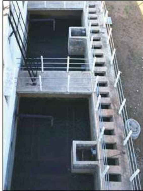
Figure 8.45: Filter Inlet Channel and Inlet Weir with Chambers
