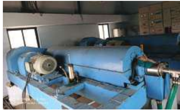
Figure 8.51: Centrifuges located on the First Floor
