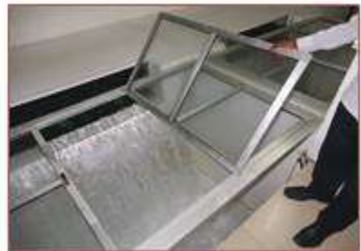
Figure 8.47: Filter outlet chamber with weir, Weir Crest Located above Top of the Media
