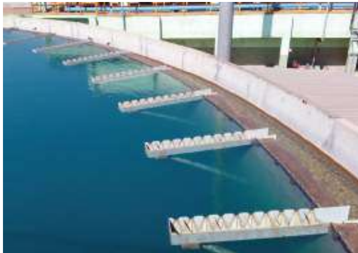
Figure 8.19: Finger weirs for Large Diameter Clarifiers/ Clariflocculators in case they exceed weir loading
