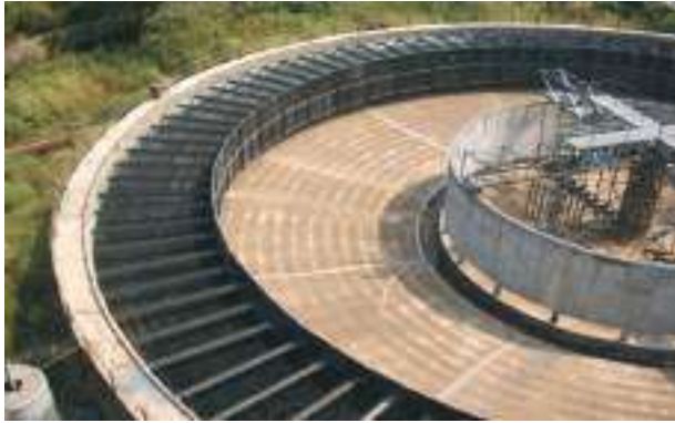
Figure 8.56: Tube Modules installed in Clariflocculator
