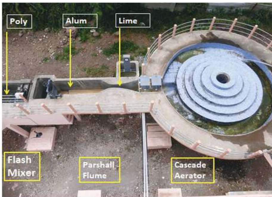
Figure 8.4: Dosing point locations in the WTP with Flash Mixer
