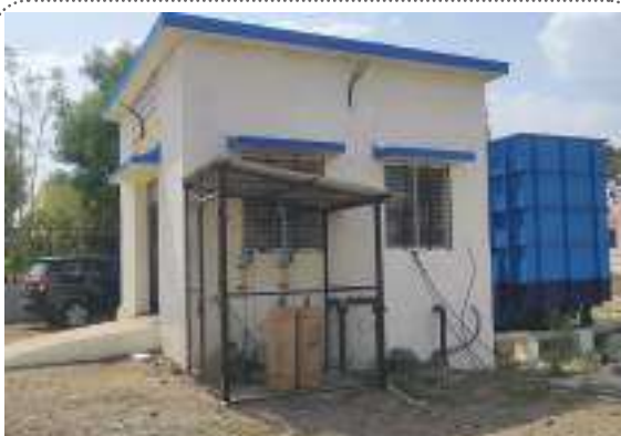
Figure 9.7: Installation of chlorine cylinders (100 kg) and chlorinators At Packaged water treatment plant, Rajapur, Dist. Ahemadnagar, Maharashtra
