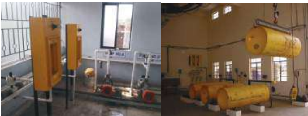
Figure 9.5: Chlorinators (Vacuum Type), booster pumps, Tonner handling in Maharashtra
