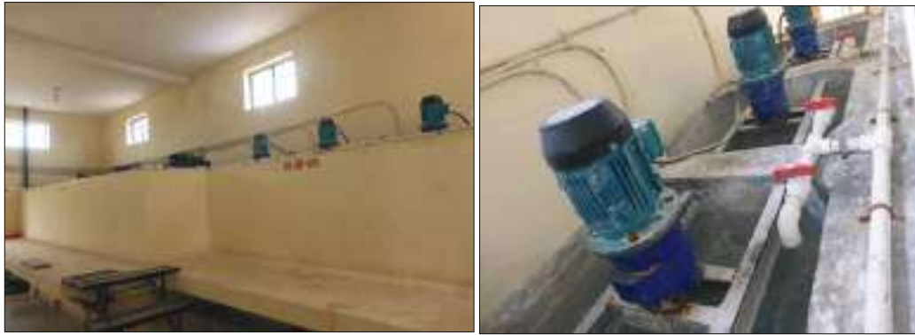
Figure 9.10: Bleaching Powder dosing tanks at 10 MLD Vaijapur WTP, Maharashtra
