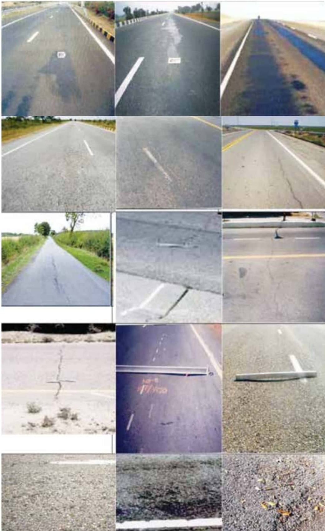
Annexe 12.1. Photographs of Distress on Flexible Pavements
