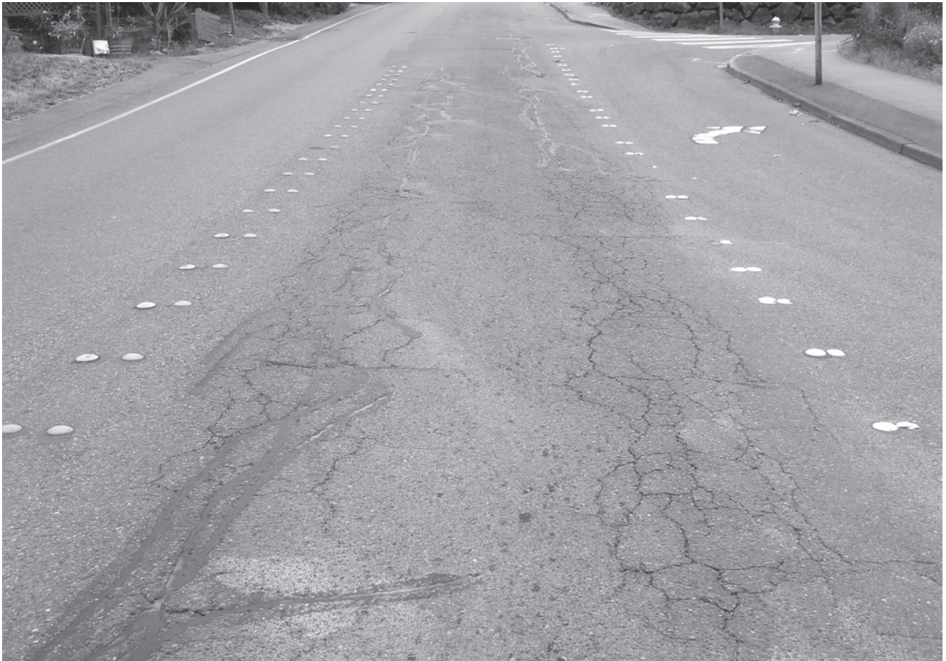
FIGURE 2.5 Fatigue (Alligator) Cracking
