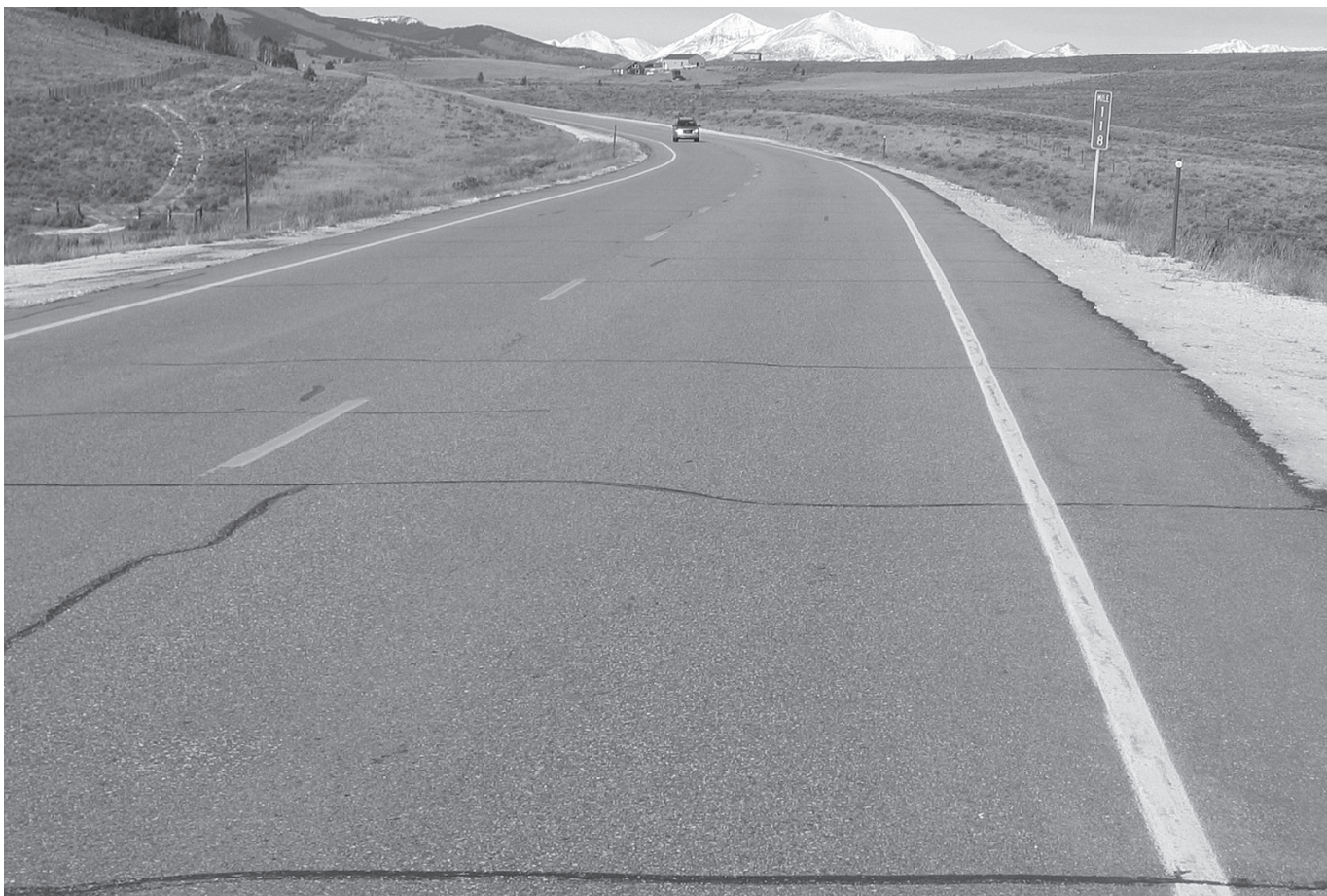
FIGURE 10.18 Transverse (Thermal) Cracking
